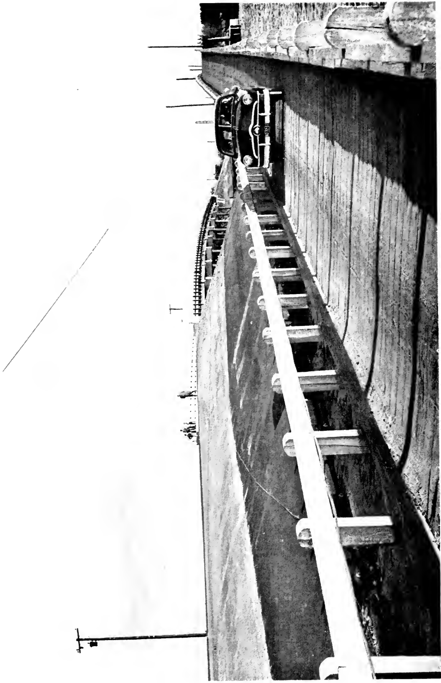
Old and new bridges at St. George's Island, Md. Route 249 in St. Mary's County.
